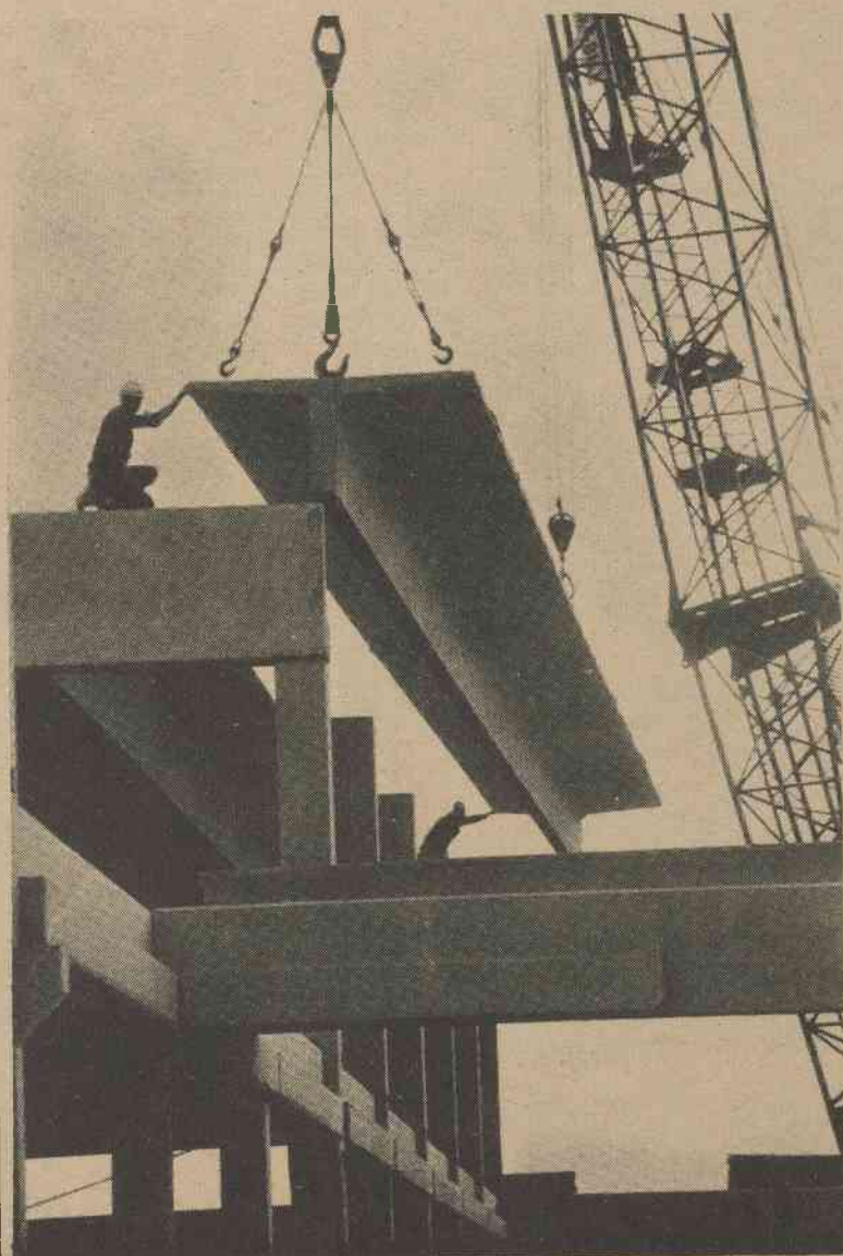
The gymnasium is slowly becoming a reality as laborers are nearing completion of the outside of the building.
