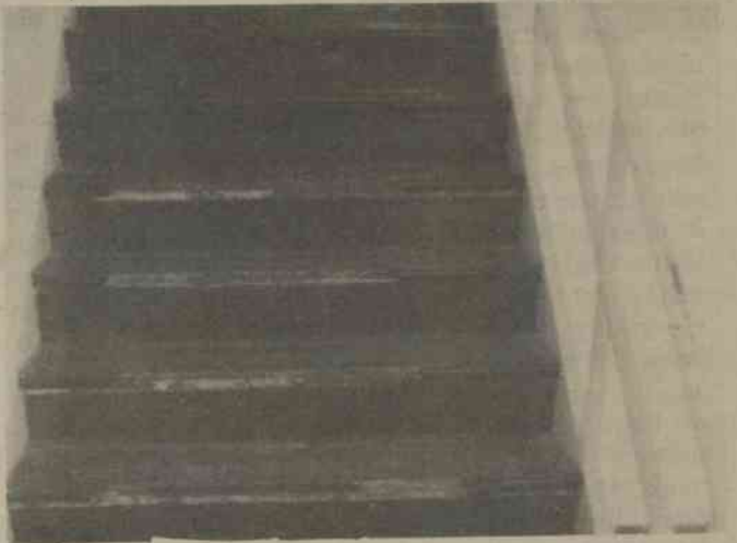
Meck dorm's lack of renovation
