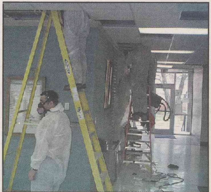
Construction crew working on wiring in Johnson Hall where asbestos was detected.
