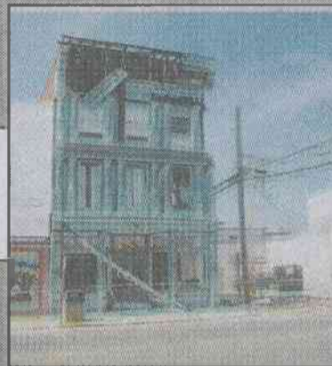
Historical building loses bricks and part of its facade during Isabel.
