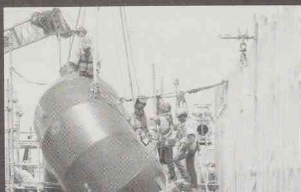
ABOVE PHOTOS: Construction workers install large water pumps along the 17th Street Canal in New Orleans, Louisiana in an effort to help prevent flooding during future storms.
