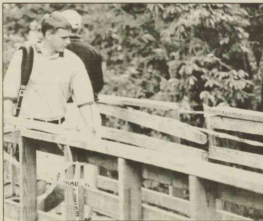
The bridge in front of the Player Golf and Tennis Learning Center received damage from a tree blown down by Bonnie's high winds.
