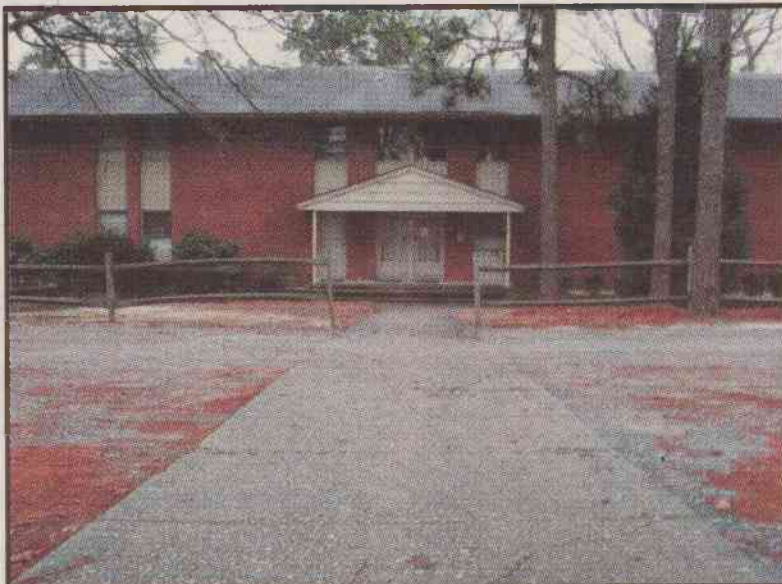
Above: The 45 year old Pines Apartments pictured from the outside. Left: one of the finger print door decoders hanging on the paint chipped outer wall.
