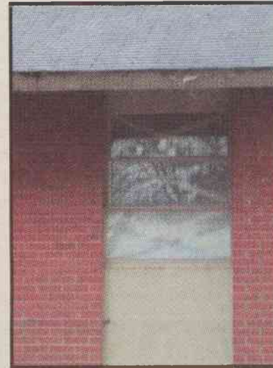
Above: The worn roof trimming on the left side of the Pines apartment
