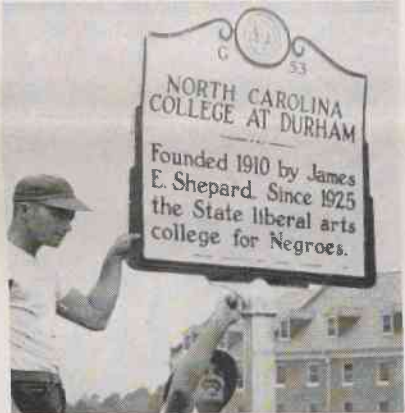
Workmen from State Highway Commission's historical marker section erect memorial to NCC's founder, the late Dr. James E. Shepard.
