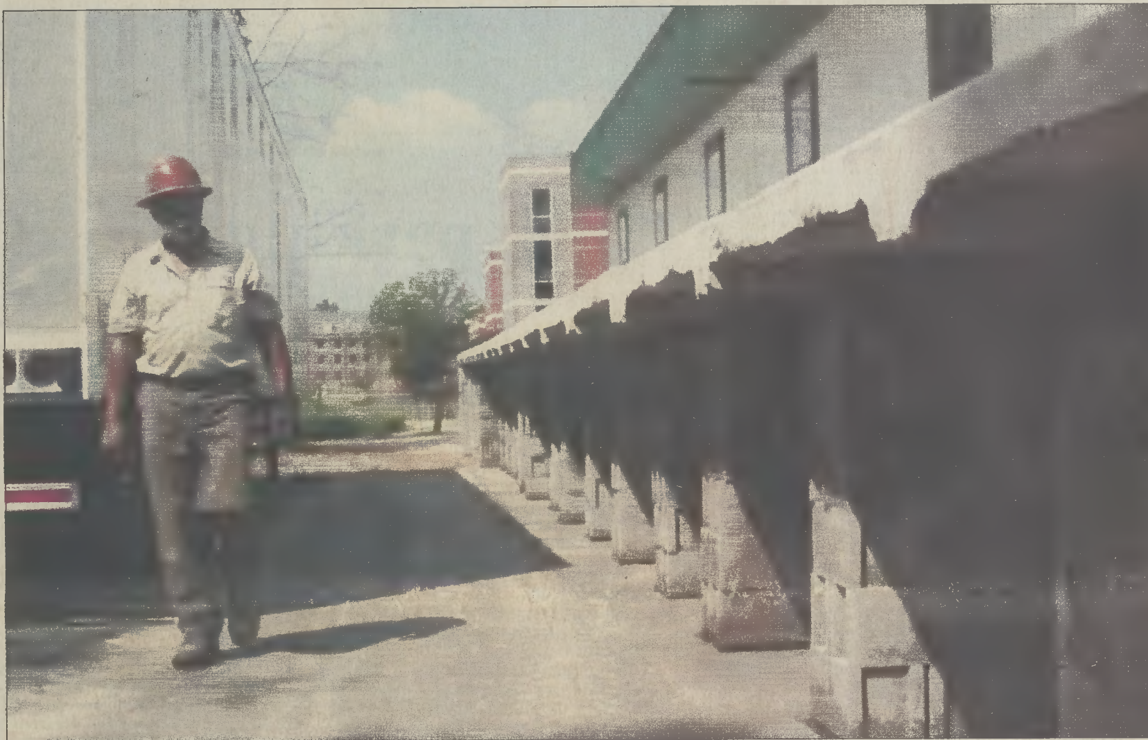
A worker walks along the installation of modular units located off Alston Avenue east of Childley Residence Annex. The units will serve as a temporary replacement for Pearson Cafeteria beginning Oct 24.
