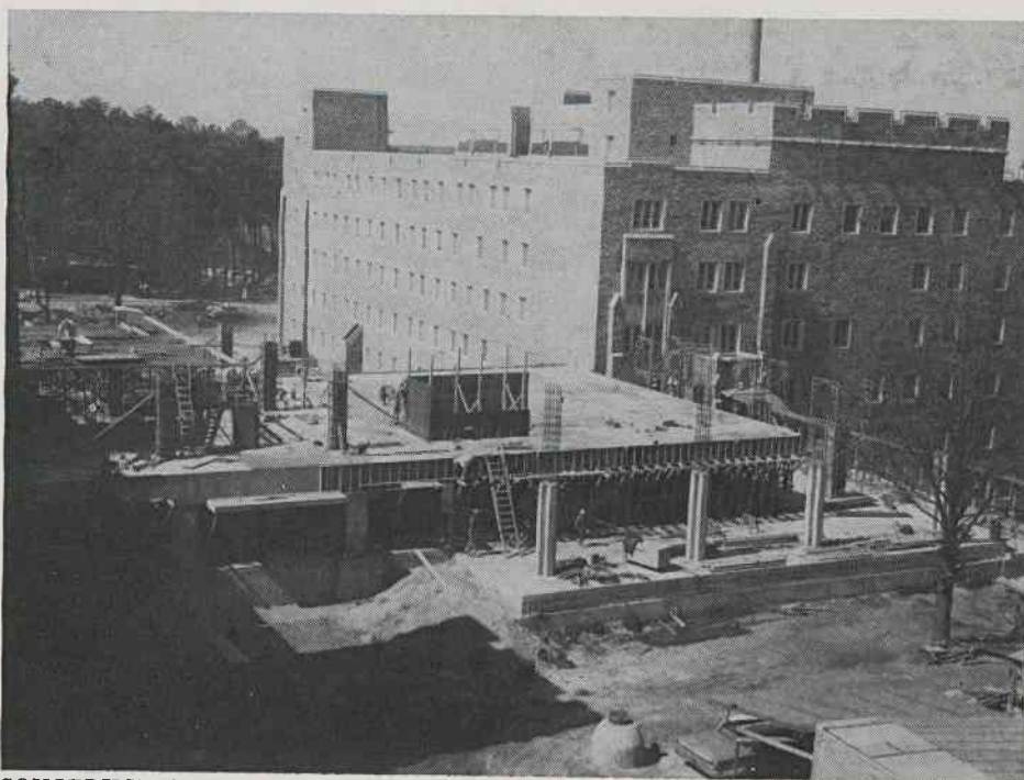
CONSTRUCTION CONTINUES ON THE NEW MAIN ENTRANCE BUILDING. —This picture of the construction, taken by Medical Illustration artist, Bob Blake, on March 18, reveals how much progress has been made since the picture was taken. Since March 18, the skeleton of the second story has gone up, and work has begun on the third. It won't be long now!
