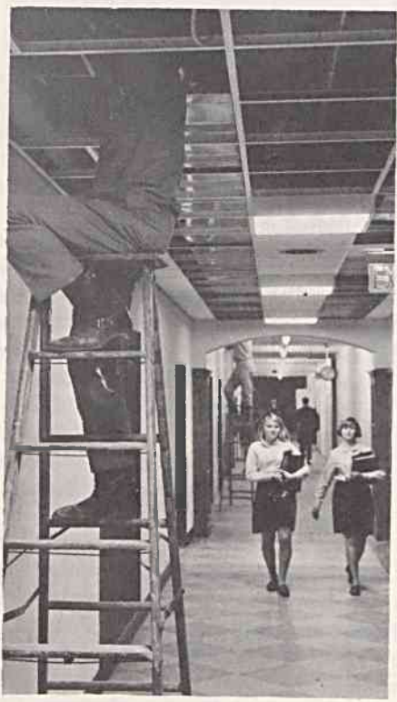
CHAPLAIN'S SERVICE —Hospital workmen install air conditioning for the new family room and hospital hostess office on the first floor near the main lobby. (Photo by Tom Knight)
