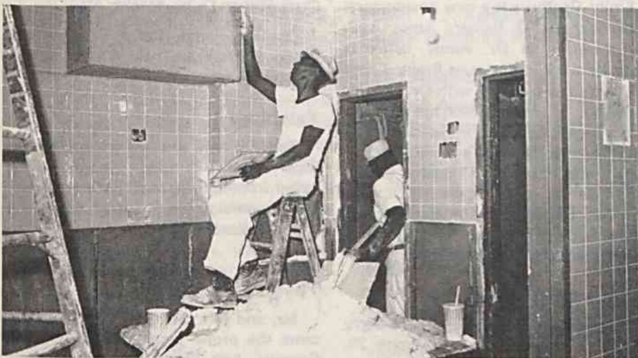
RENOVATION --Workmen are busy renovating four operating rooms to bring the total in the Duke OR suite to 18. (photo by Bill Boyarsky)
