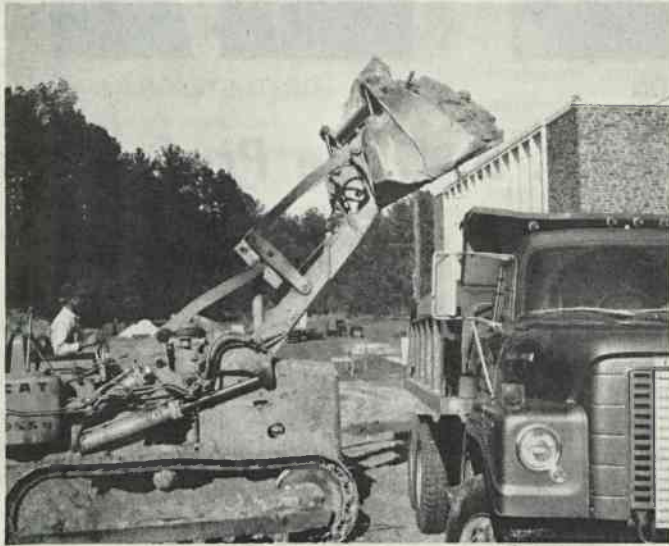
CONSTRUCTION UNDERWAY —Workmen broke ground in March for Duke's newest building, a research facility named for the late Alexander H. Sands, Jr. Mr. Sands was one of the original trustees of the Duke Endowment. (staff photo)
