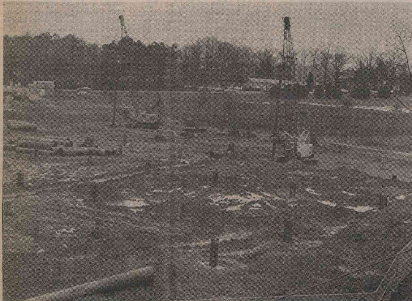
HEIGH-HO AND UP SHE RISES—On Monday, heavy rains put the damper on construction of Duke North, turning the ground into a quagmire of shoe-sopping mud. Evidenced by this photograph, progress is being made, however, as steel forms of reinforced caissons show themselves above the
