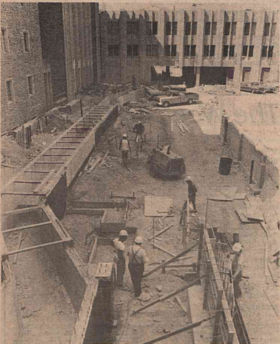
LOOKING NORTH—Workmen lay the foundation for a lobby which will be the south terminal of the PRT (Personal Rapid Transit), linking Duke Hospital South and Duke Hospital North. The photo, taken above the present emergency entrance, shows the tunnels through which the two PRT cars will pass under the Edwin A. Morris Clinical
