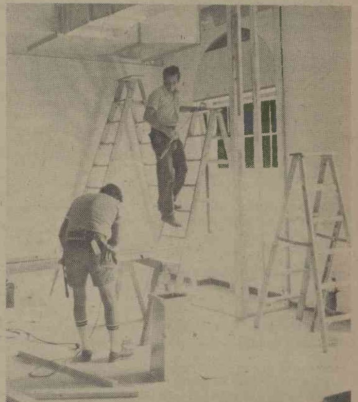
Workmen continue renovations of Mooney first floor through day and night for early completion.
