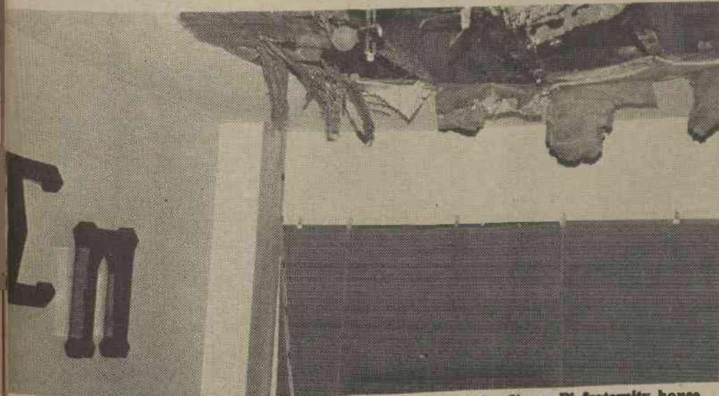
CAVE IN—Due to leaking pipes, the once sagging ceiling of the Sigma Pi fraternity house became a large, gaping hole last week. Photo by Nader Hamidpour.
