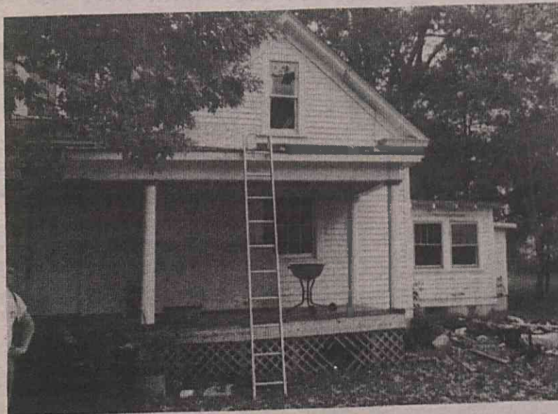
This residence, located at 301 Haggard Avenue, has been abandoned since the fire.
