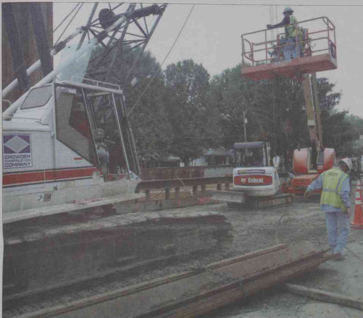
Workers from Crowder Construction Company secure steel beams into the ground using compression machinery. Excavating the tunnel has been a noisy process that has resulted in three students who live close to the site being moved to temporary university housing.
