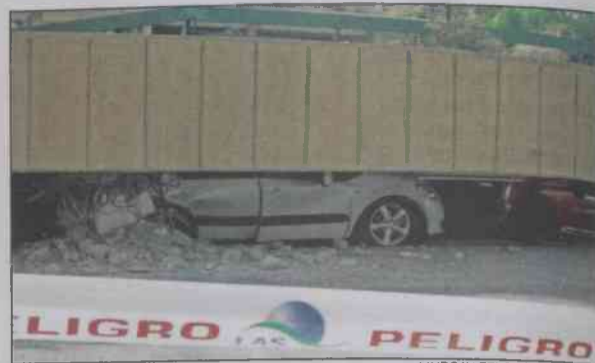
LINDSAY FENDT | Photographer The ceiling of a parking garage in a Santiago neighborhood collapsed during the earthquake. The 56 cars that were inside the garage were all damaged beyond repair, and the surrounding buildings suffered structural damage.
