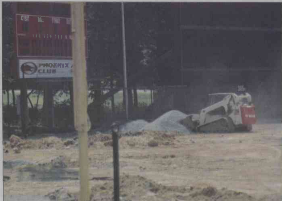
Updates to Latham Park began immediately after the final home baseball game. One part of the renovations include moving back the left field fence and raising it to a 12-foot fence.
