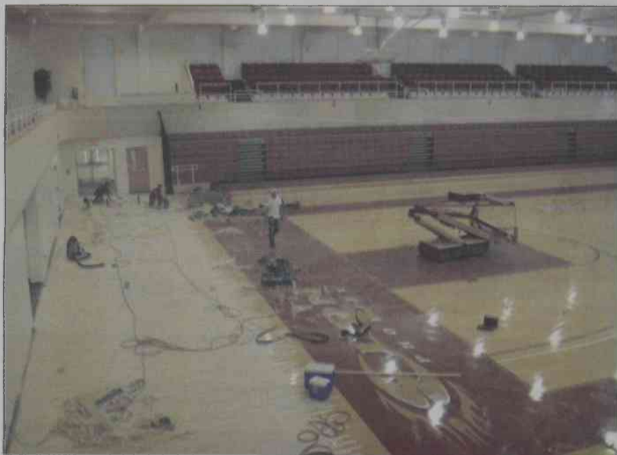
Phase one of the Alumni Gym renovations began June 11. The first steps of the renovation include replacing the flooring of the gym. The renovations are expected to be finished in mid-September.
