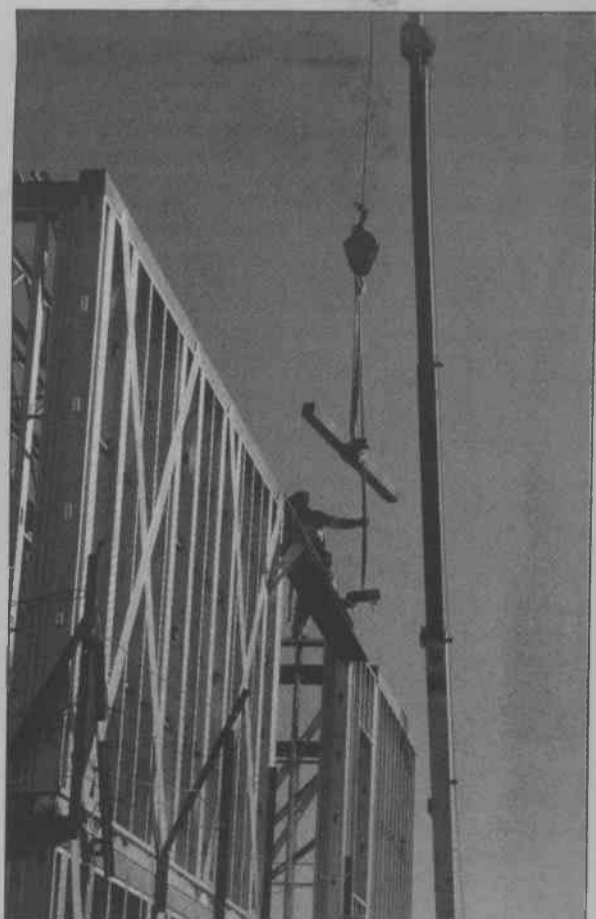
The construction site for the future Colonnades dorms. JULIA MURPHY | Staff Photographer
