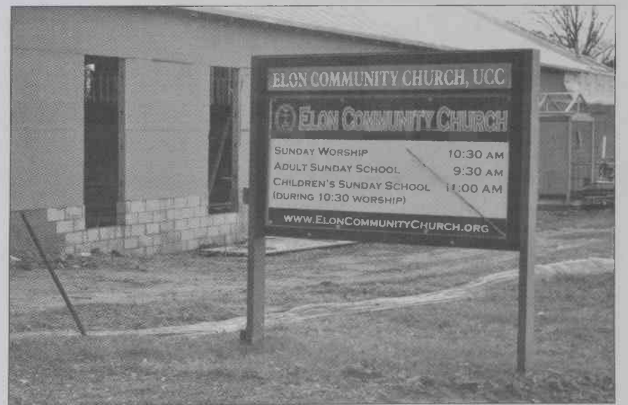
Officials at the Elon Community Church hope to have the expansion of their facilities completed in time for Easter Sunday next year. Construction was delayed but is now back on track. ELIZABETH EVERETT | Staff Photographer
