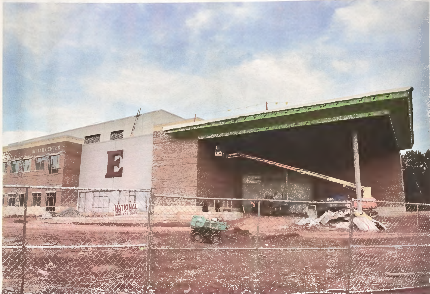
Construction continues on Schar Center as workers put finishing touches on the exterior while the weather is nice. The new center will seat 5,400 people and will be the future home for Elon athletics.
