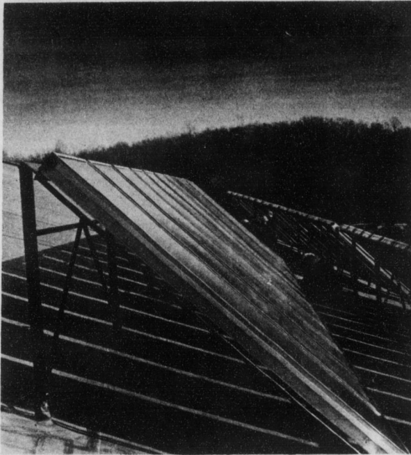
The gym has progressed since this picture of the solar panels was taken, but who gets to use it when it's done is still a matter of concern.
