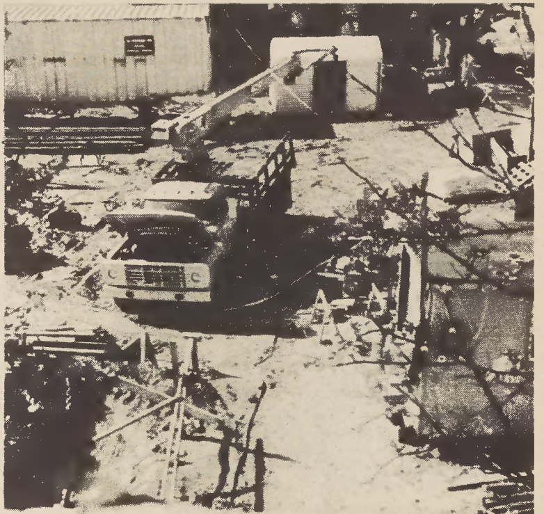
The construction at Salem's library continues week after week. This particular corner will one day boast a reconstructed Moravian house.
