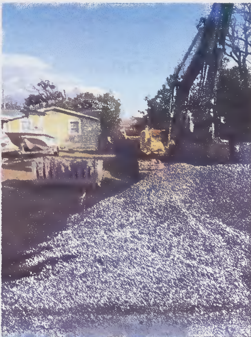
Stormwater line being installed, looking east from Juniper Road—Photo by Brian Kramer
