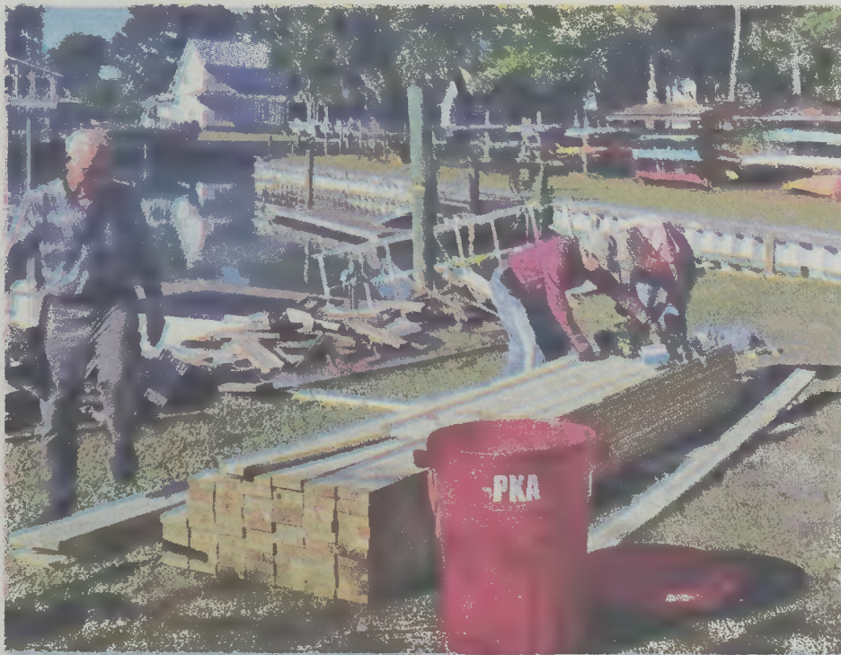
From left, Ron Huggler, Dick Belanger and Darlene Sanchez working to resurface and reinforce the east dock at Brock Basin.—Photo by Robert Cox
