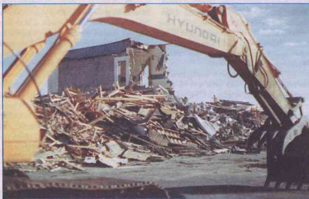
Etched against the sky, a remnant of the Iron Steamer Motel is framed by the arm of an excavator being used to tear it down.
