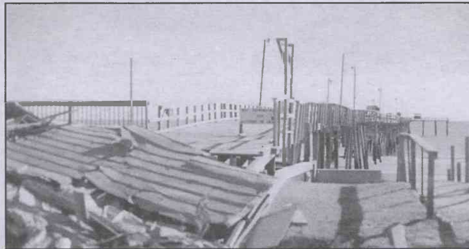
With the pier house already reduced to rubble (foreground), the Iron Steamer Pier itself awaits the attention of demolition crews.
