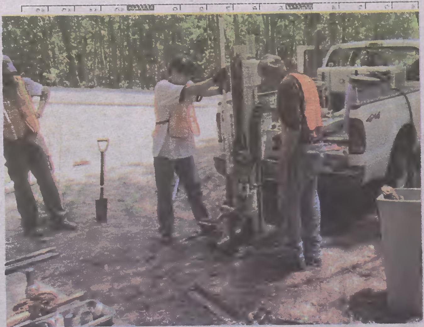
Researchers from East Carolina University installing a groundwater monitoring well in 2015 using a "geoprobe" drill rig.—Photo courtesy of Dr. Alex Manda
