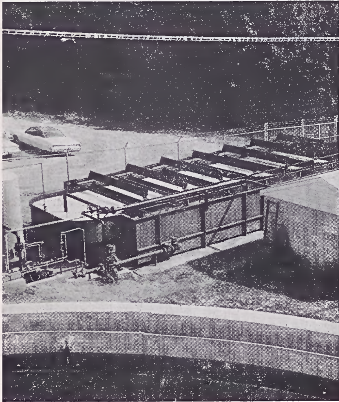
Favir unit uses air flotation to separate oil particles from water. Sludge collected by skimmers will be incinerated. Water goes on to two lagoons where aeration takes place.
