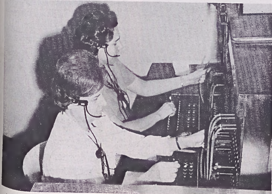
BUSY HANDS of Elaine Cox (foreground) and Marie Murray manipulate switchboard at General Offices, Eden. These operators use good telephone manners. How about you? Have you ever thought about the impression you create over the telephone? For hints on good telephone manners and procedures, see story on page three.
