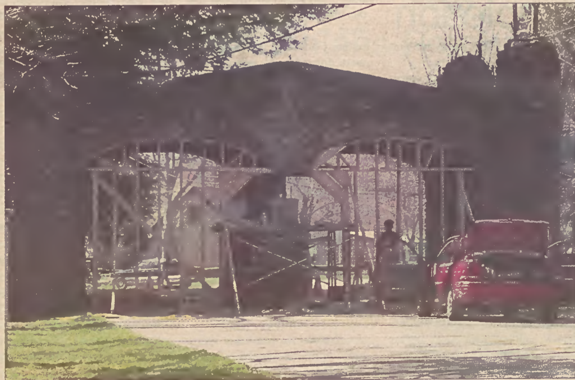
A long-time symbol of Montreat, the gate is currently undergoing repairs from a recent accident. Repairs should be complete by April 1, 2003
