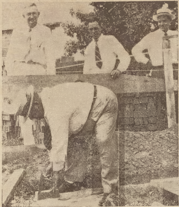
FIRST BRICK—Legionnaire W. Luther Etheridge is shown laying the first brick of the $20,000 Community Building, sponsored by the Selma Post No. 141, American Legion. Others in the picture, left to right, are Dr. E. N. Booker, Ed Creech and Wade Hicks.
