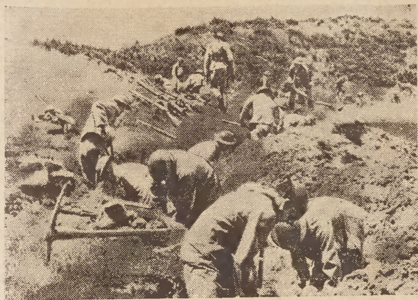
For obvious reasons, the exact location of these trenches in New Zealand can not be given. The island is erecting extensive and effective defenses in readiness for the invading Nipponese.
