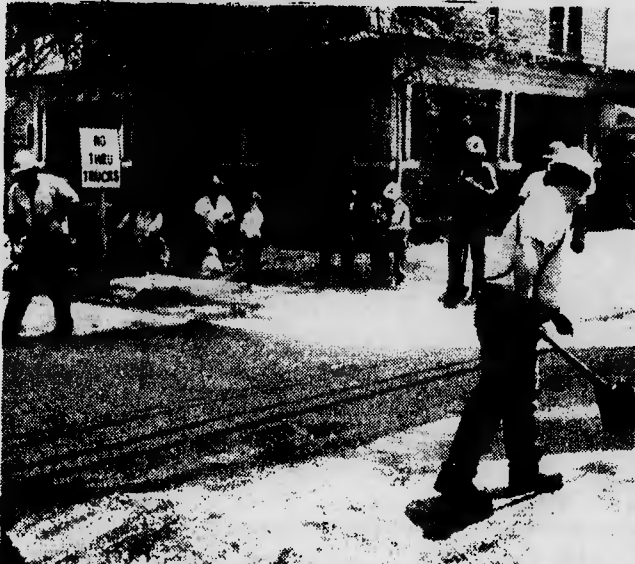
Main Street in Vanceboro was buzzing with activity last week as it got a much needed new cover.
