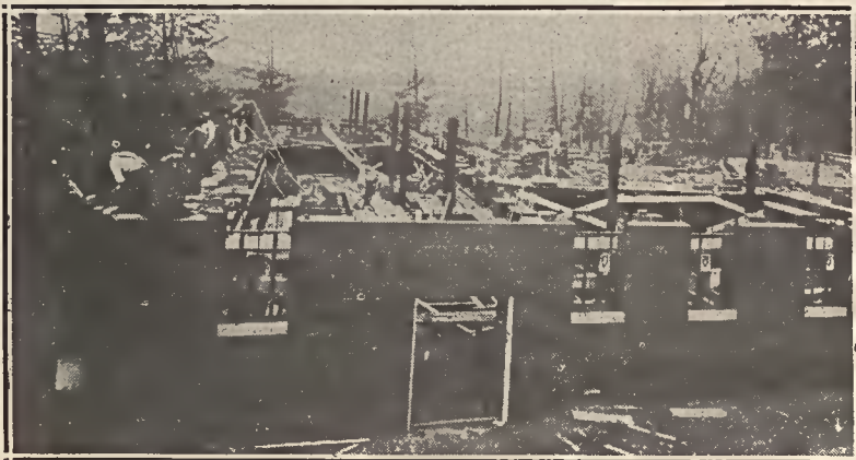
Picture shows progress being made on the Edna Corpening Moore Dormitory being erected on the hill overlooking the east campus. The contractors expect to have the walls completed by January 1.
