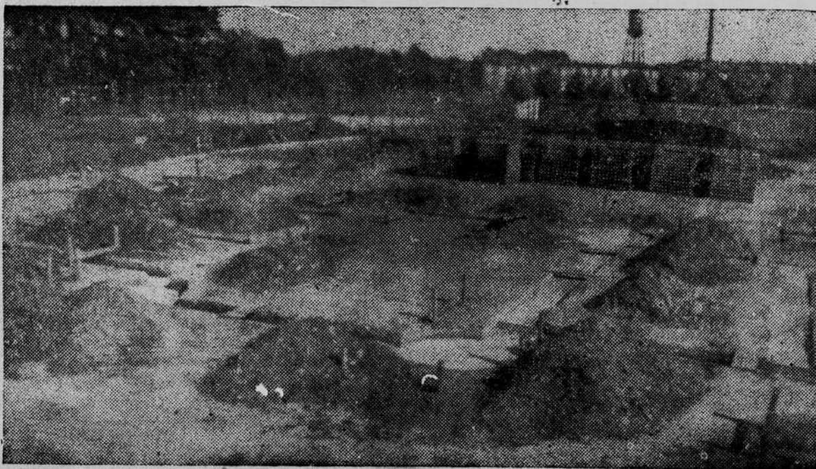
Above is a bird's-eye view of the armory site at the corner of Ninth and Hamilton Streets. The concrete foundation is practically finished. Work progresses on the building according to schedule, it is said.
