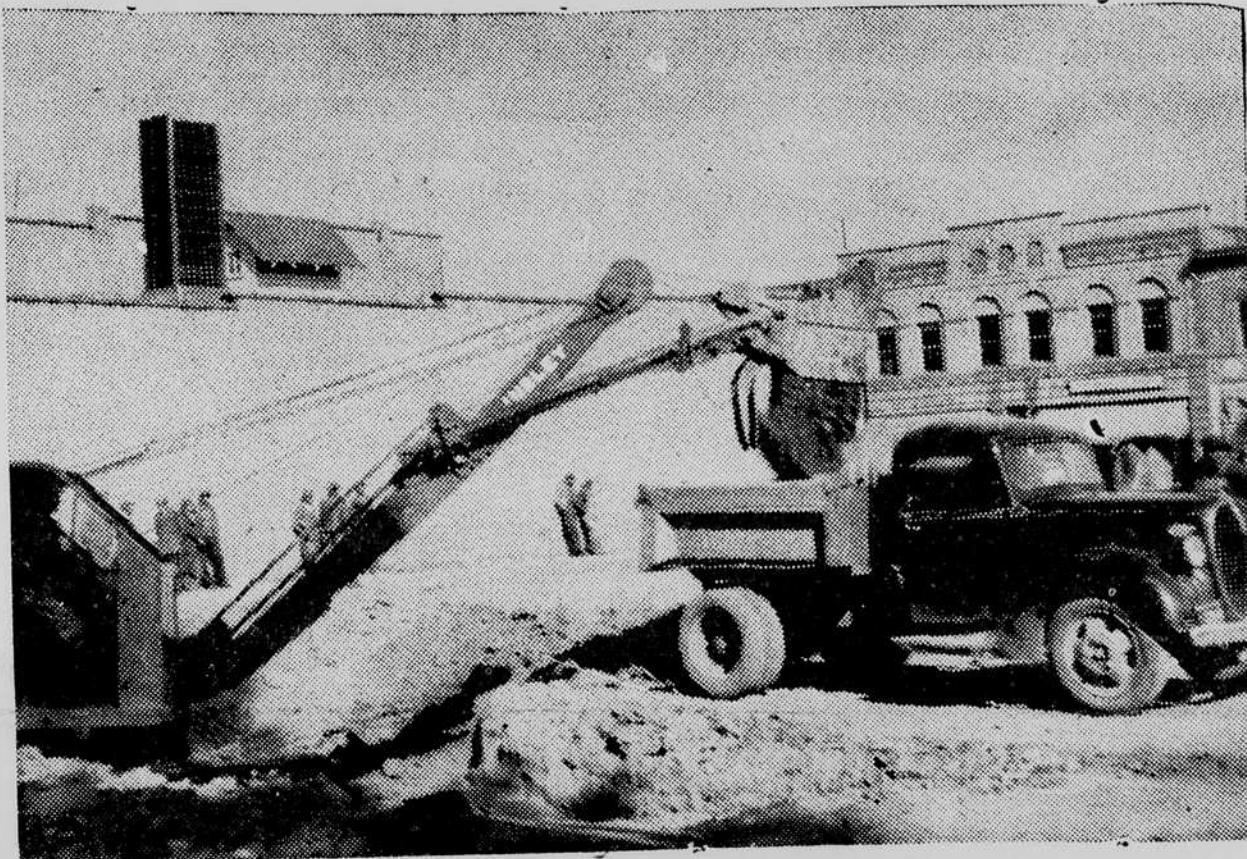
Hundreds of interested spectators daily watch the big power shovel, pictured above, as it excavates for the basement of the building soon to be occupied by the J. C. Penny Co. on Roanoke Avenue, actual construction of which started this week.
