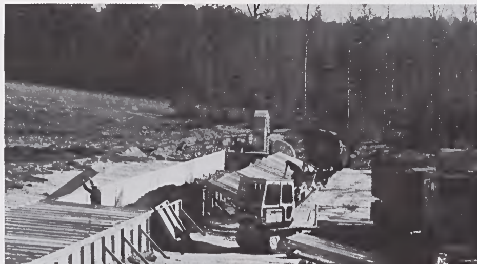
FIRST LOAD: Arnold Morgan loads the waiting truck as Conley Mathis removes roof panels. When all the dried sludge has been removed, the bins will be filled again and the roof sections reinstalled for the next load.
