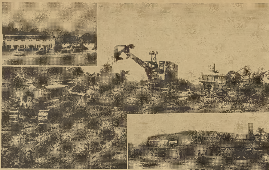
The new gym has gone from the mud bog in the middle of the picture to the beams in the bottom. This skeleton just may get a covering by May, in time for graduation.
