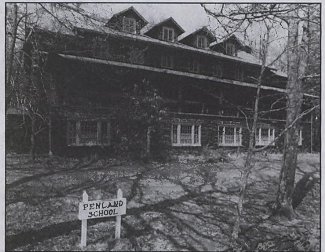
The Craft House will have a major renovation this winter supported with gifts from Friends of Penland
