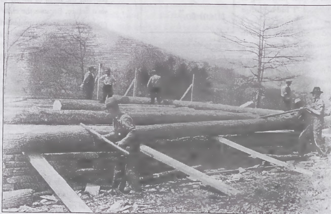
Allegedly the largest log structure in North Carolina, the Craft House was named for Edward F. Worst, who was one of the country's leading experts on hand weaving. His weaving "institutes" attracted the first craft students to the mountain. Today the building accommodates the coffee house, the school store, the library, and two floors of student housing.
