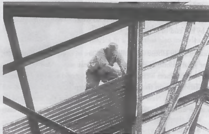
Even a large steel building gets put together by hand. Contractor Paul Convery is fastening roof panels with a powder-activated nail gun.
