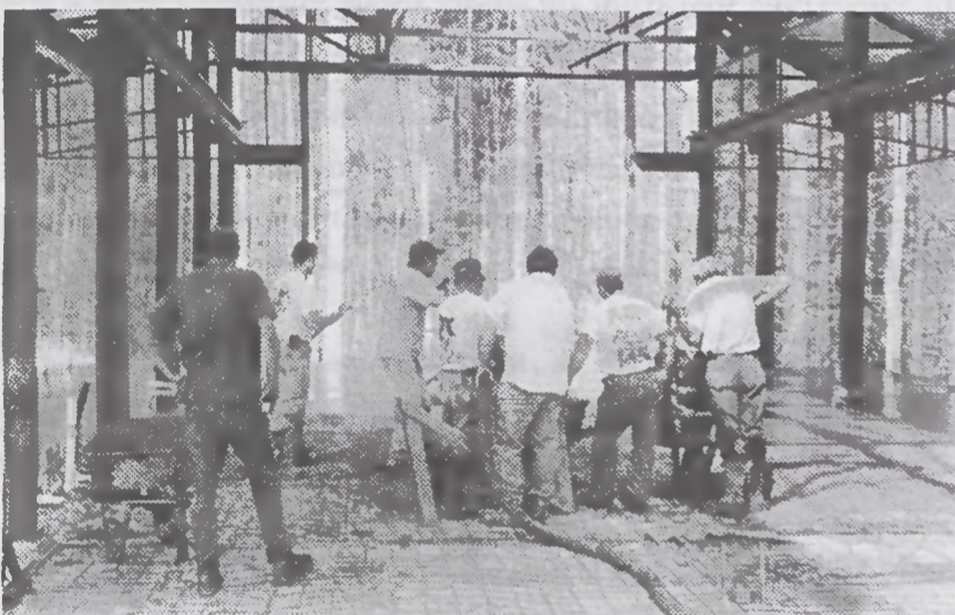
One hundred and three yards of concrete; let's see that will take about fifteen mixer trucks, a concrete pump, a big crew, and a very long day.
