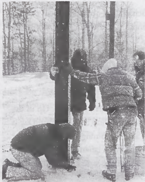
Headless of the weather, Appalachian Building Services began assembly the day the steel components were delivered.
