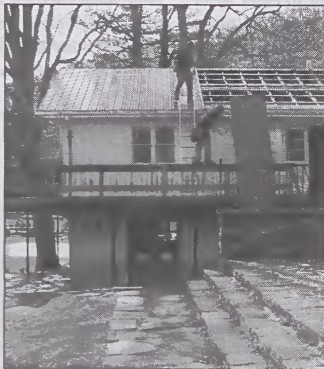
The metals studio got a new roof this April: just one of the studio improvements financed by the campaign.
