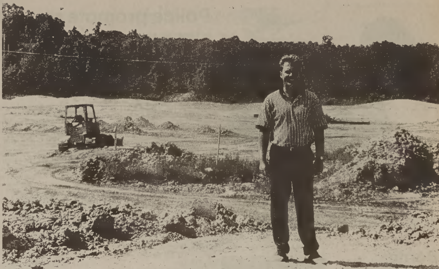
UNDER CONSTRUCTION —Jeff Guman, golf professional at Prestonwood, stands atop a small mountain of dirt which over-
