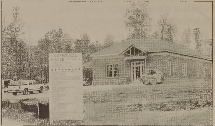
ONGOING CONSTRUCTION—Work on the town's police station is several weeks behind schedule. The board is considering whether to charge the contractor a penalty for the delay.
