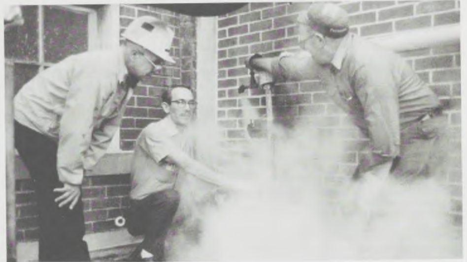
BEFORE, TRAP LOSING STEAM – This steam trap, one of about 2,500 in Ecusta Paper, loses steam because it is in bad condition. A Maintenance Department program was begun and implemented several months ago to replace traps which are allowing steam to escape, and causing energy to be wasted. By plugging up steam leaks, it is estimated that in excess of $100,000 yearly will be saved, according to Jim McIlwain, Group Director of Energy Conservation. Left to right are John Hillyer, Manager of Energy Conservation, Charles Jones, Pipefitter and Vernon Jones, Welder.
