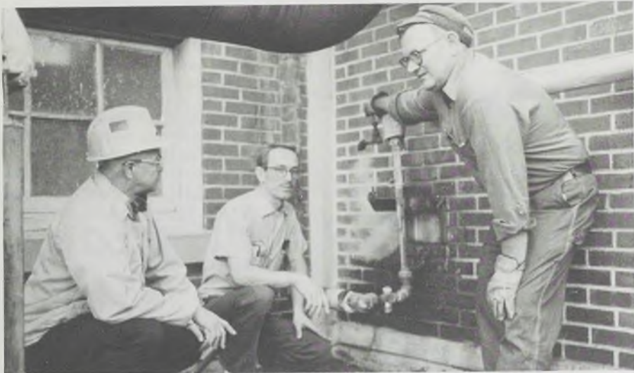
AFTER, ENERGY EFFICIENT STEAM TRAP – One of 2,500 Ecusta Paper steam traps, this one no longer allows steam to be lost. By reconditioning it, energy is saved as well as substantial annual dollars. Part of a Maintenance Department project to put all steam traps in first class condition, the program was implemented several months ago and has been dubbed by Olin officials as Ecusta Paper's North Slope discovery. Left to right are Manager of Energy Conservation John Hillyer, Pipefitter Charles Jones and Welder Vernon Jones.
