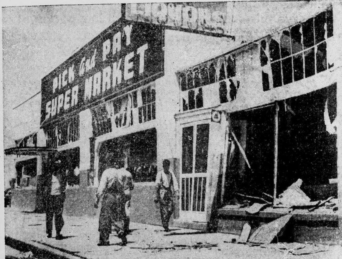
BUILDINGS DAMAGED miles from Texas blast scene—Although located miles from the scene of the Texas City, Tex., explosions these two stores were badly damaged by the shock. Windows were shattered and sections of the framework buckled.—(International Soundphoto).
